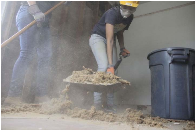
Sophomore Jackie Medina shovels insulation at a Habitat for Humanity renovation. Photo courtesy of Harold Pierce, The Californian .
